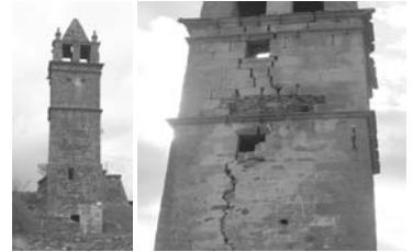
Figure 1: Mogadouro Clock Tower: general view and severe damage before rehabilitation
