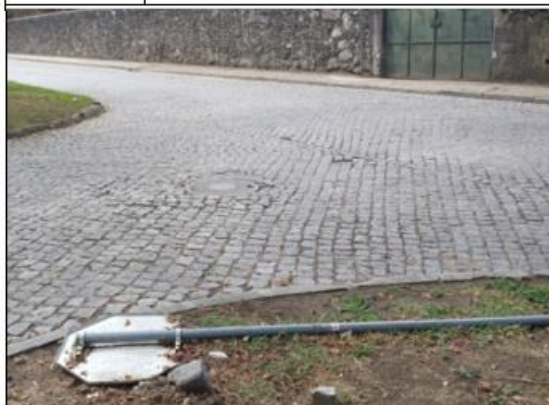
TRNR4 – “Sinal STOP completamente derrubado.”
