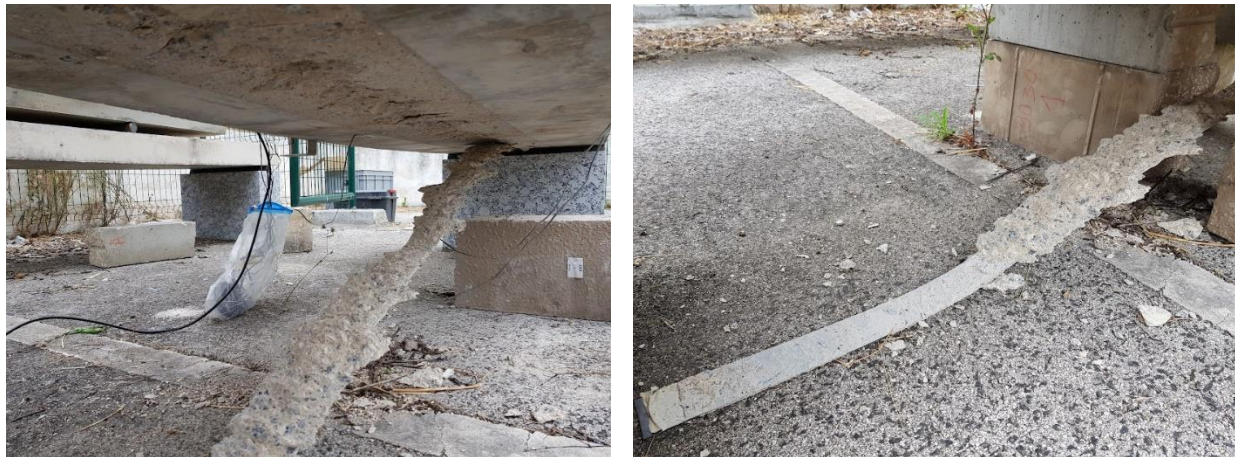
Fig. 13. CFRP detachment on GA slab of E3 environment \sim 26000 h (3 years) after loading.
