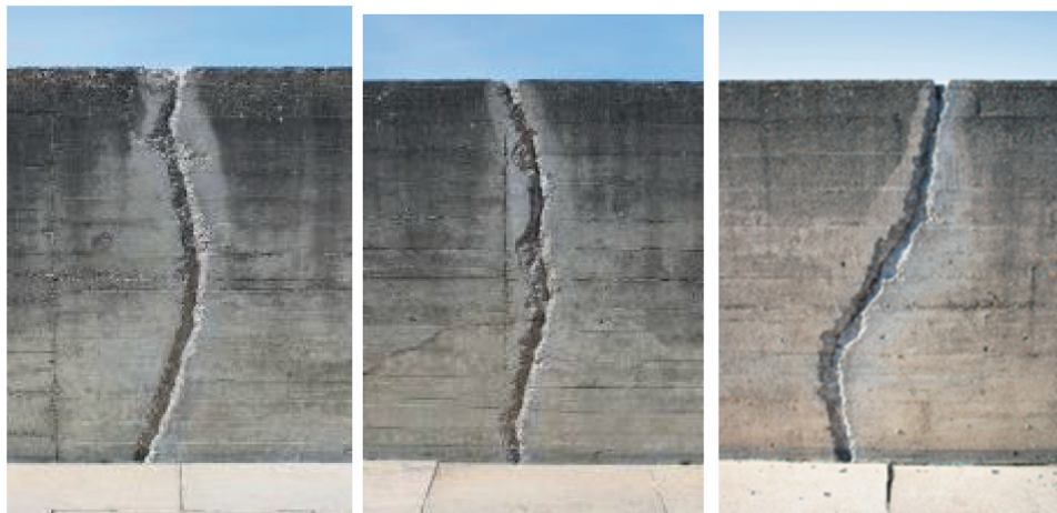
Figure 21. Vertical cracks due to the absence of movement joints after recent conservation by Alvaro Siza (2021).
