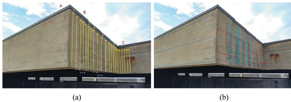
Figure 18. GPR tests on the beam over the changing rooms: (a) location of the GPR profiles; (b) likely reinforcement details of the connection between the beam supported by the two cantilever beams.
