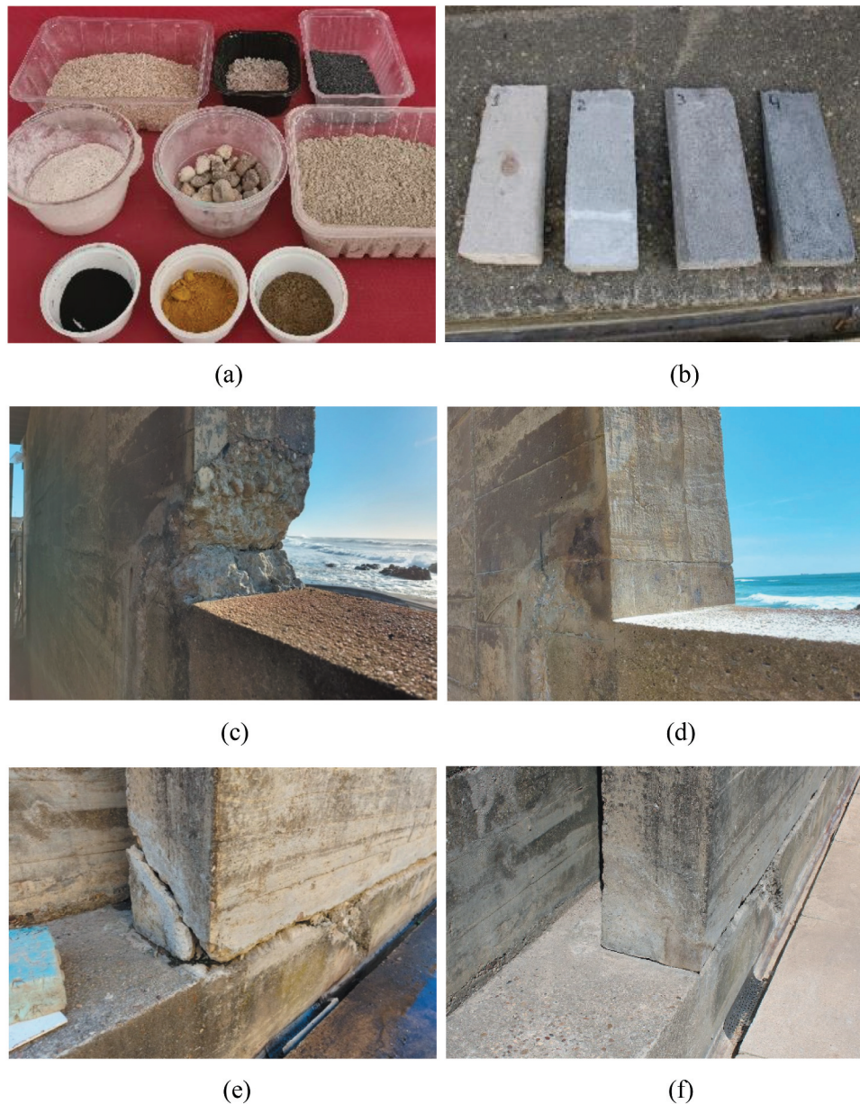
Figure 20. Pilot demonstration of concrete repair: a) Aggregates and pigments for repair mortar; b) Samples for concrete repair (4 of 10); c) R1 before and d) after concrete repair; e) R2 before and f) after concrete repair.
