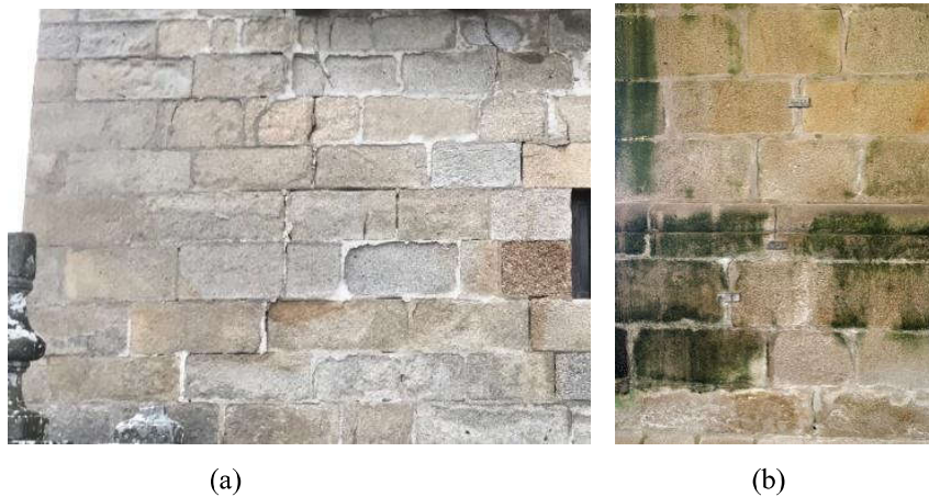
Figure 2: Cracks under the balcony of the tower in (a) external west facade and (b) internal east facade.
