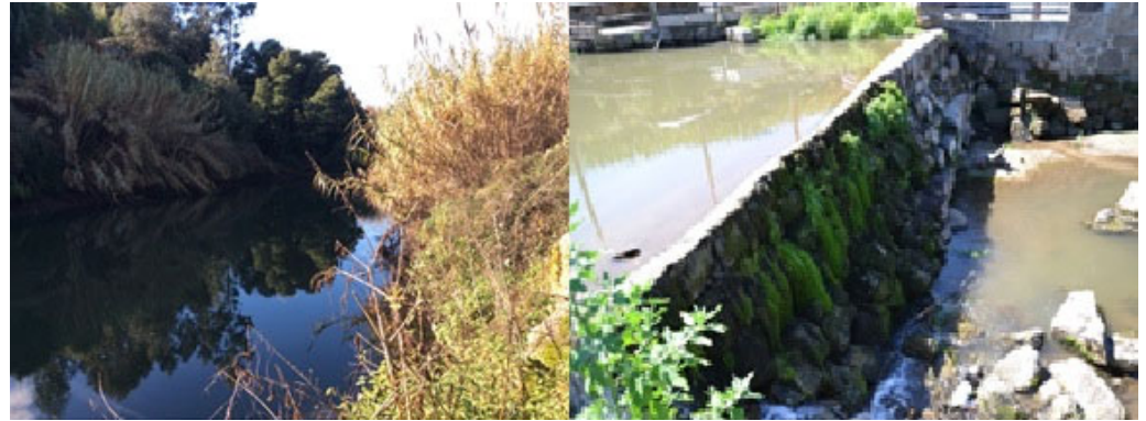
Figure 7. Backwater effects, revealing environmental impacts, and incapacity of transposition by fish species (nos. 38 and 16).
