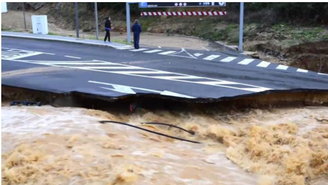
Figure 55. Flood damage and service disruption of road the Algarve region in Portugal. Photo: Sky News ( https://news.sky.com/story/one-dead-as-severe-flooding-hits-portugal-10341035 )
