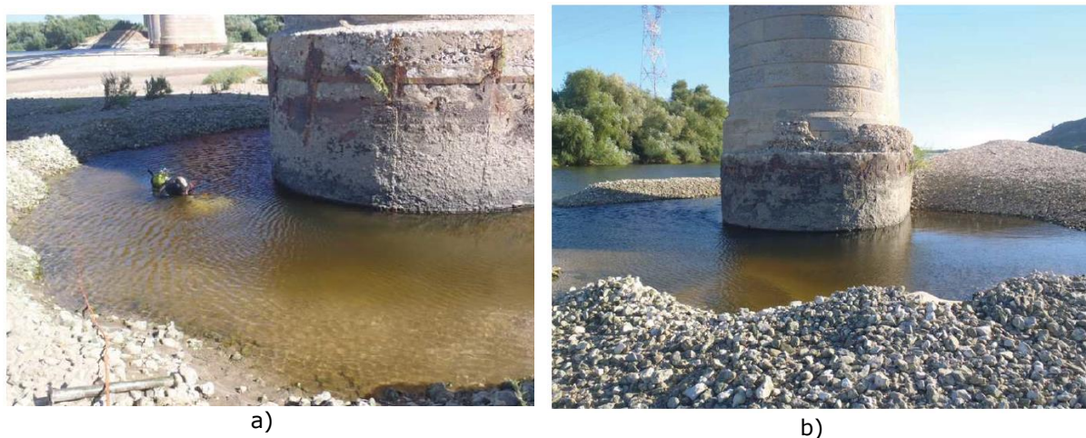
Figure 33. Presence of local scour in bridges within Class III
