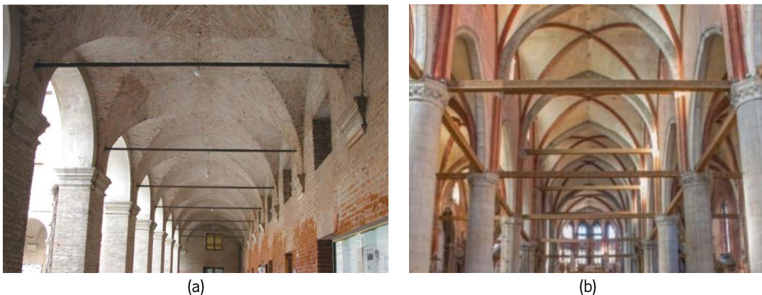
Figure 1-14. Ties applications: (a) steel ties in the cloister of Complesso dei Tolentini, Venice (Italy), (b) wooden ties / struts in Santa Maria dei Frari Church, Venice (Italy) (Bussi, 2011).
