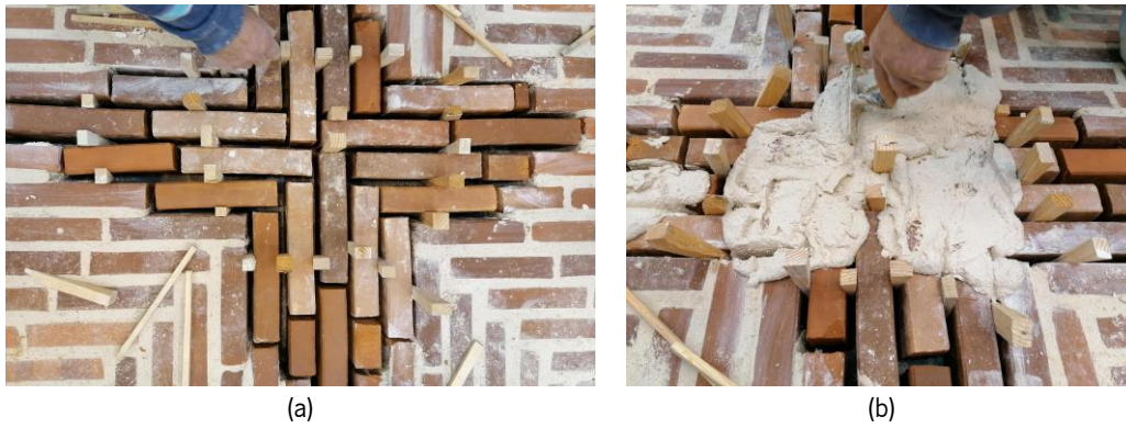
Figure 5-8. Closing the key of the vault: (a) disposition of the bricks with their misalignments, (b) filling the joints.
