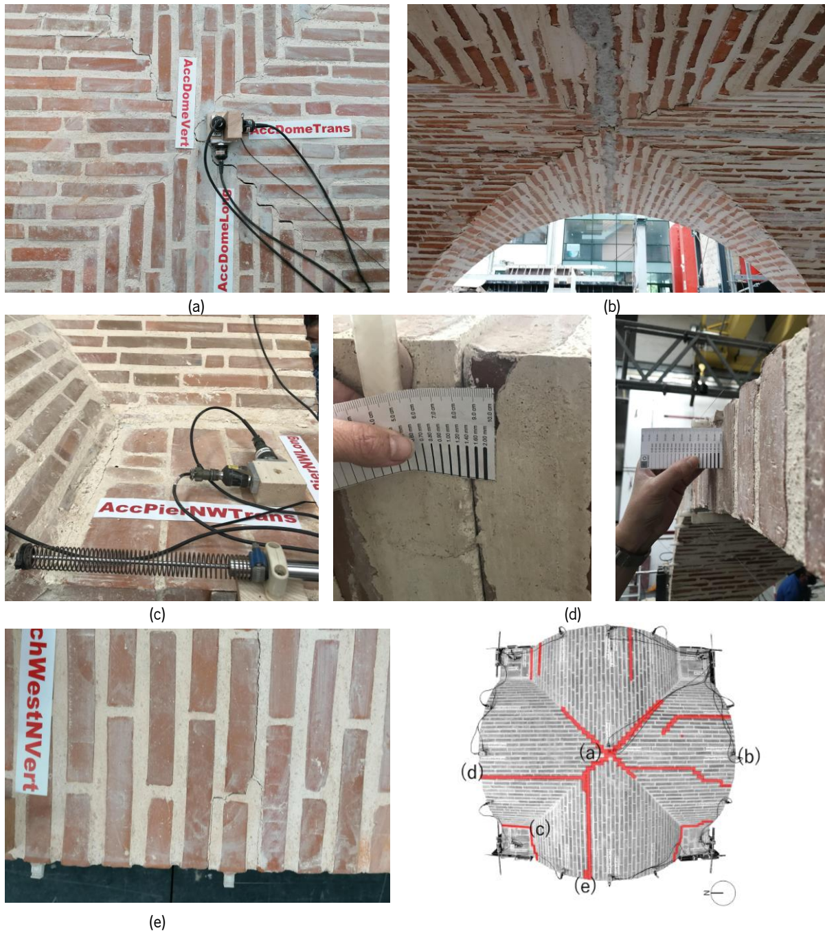
Figure 6-7. Details of the damage for the unstrengthened specimen after ST-UNS-75%, for (a) to (e) views.
