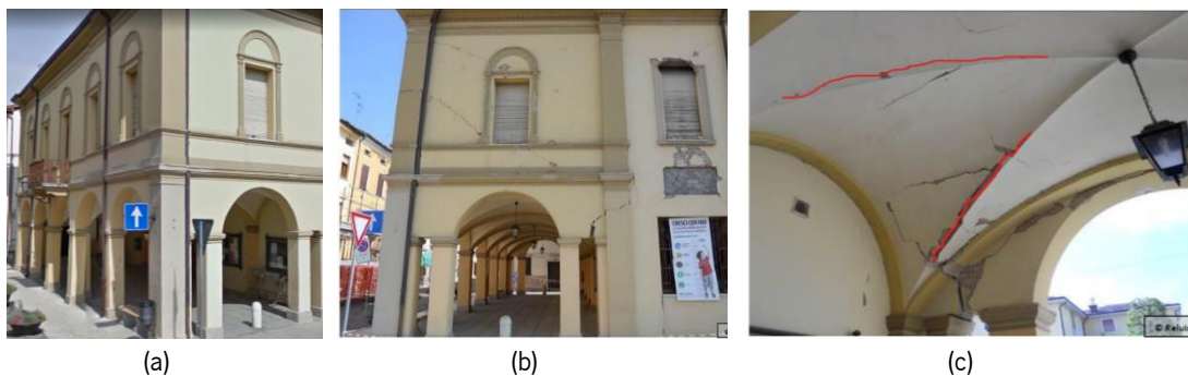
Figure 1-12. Damage on cross vaults after Emilia earthquake associated with shear behaviour: (a) undamaged view of the Town Hall in Novi di Modena, (b) shear failure of the masonry panels, (c) shear failure of the masonry cross vaults (Occhiuzzi et al. , 2012).
