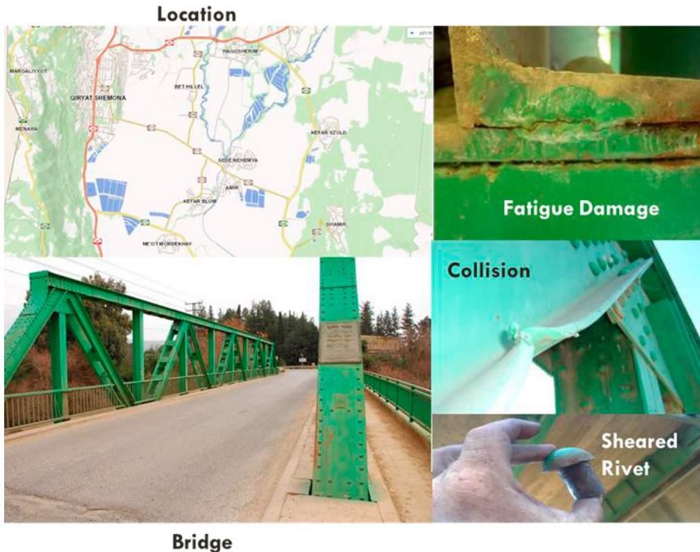
Figure 36. General information of the case study truss bridge and related damages.
