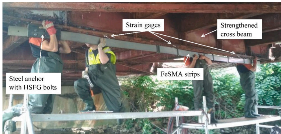
Fig. 14. Installation of the Fe-SMA plates on the lower flange of the bridge girder.
