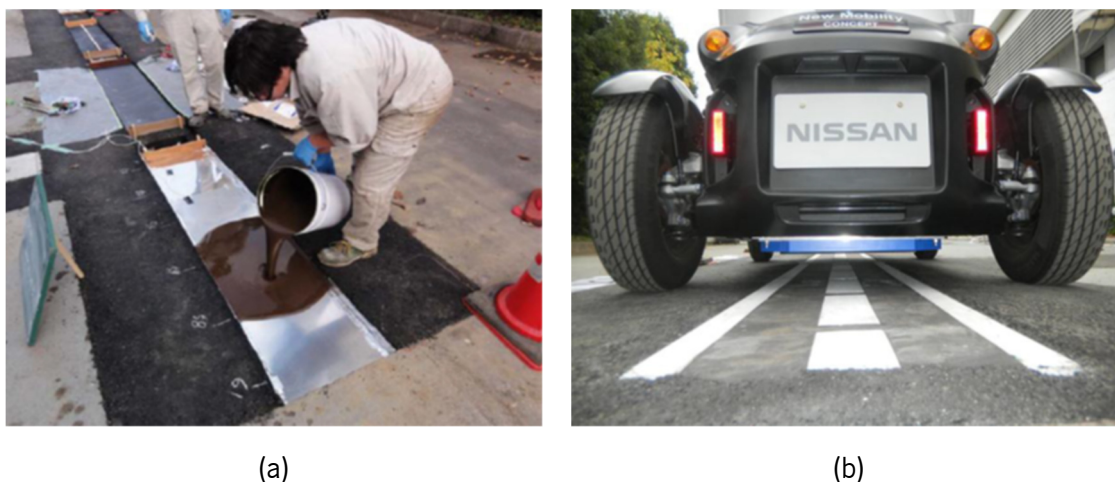
Figure 101: Nissan 1 kW prototype DIWPT lane under construction (a) and during tests, with the secondary coil installed on board of the New Mobility Concept Car (Renault Twizy). Extracted from [108].
