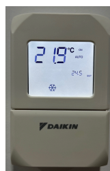
Figure 64: Fan coil thermostat.
