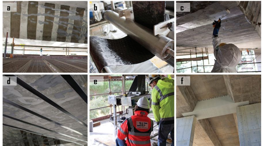
Fig. 1: Strengthening of a concrete bridge with externally bonded CFRP materials: (a) sealing of cracks; (b) pre-impregnation of CFRP sheets; (c) application of CFRP sheets; (d) EBR CFRP laminates; (e) technical inspection; and (f) finished strengthening (from Reference 65)
