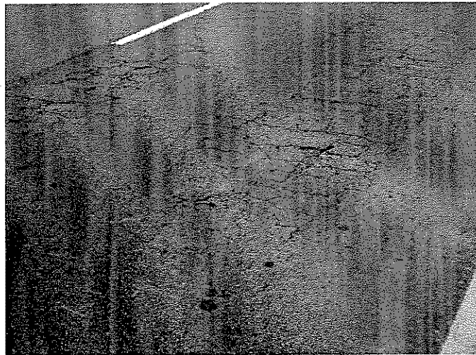
Photograph 2 – Pavement in failure condition
