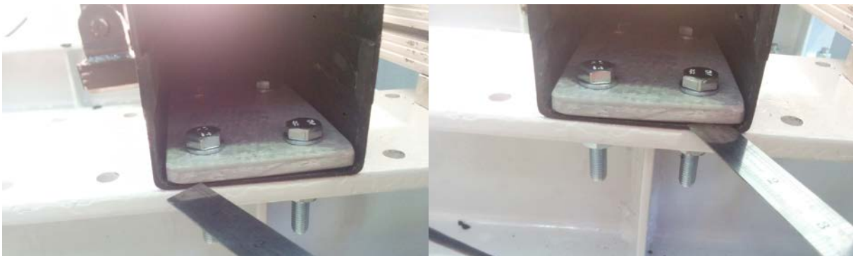
Figure 6.28 - Gap formed between the composite shell component and pultruded plate
