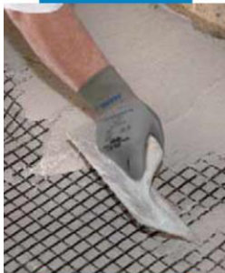
Application of the second layer of Planitop HDM Restauro by trowel on the outer face of a vaulted ceiling to cover the Mapegrid G 220 with an even coat
