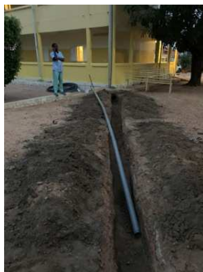
Picture #26 – Wired network pipelines to link all hospital departments
