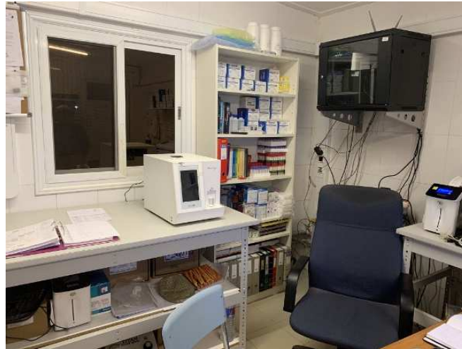
Picture #32 – Server, switches and internet router all together in same box
