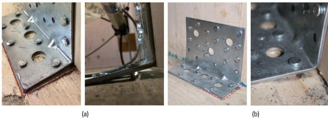
Figure 4.16 – Damages observed in the AE116 connectors between floors: (a) Monotonic transverse direction; (b) Cyclic transverse direction.
