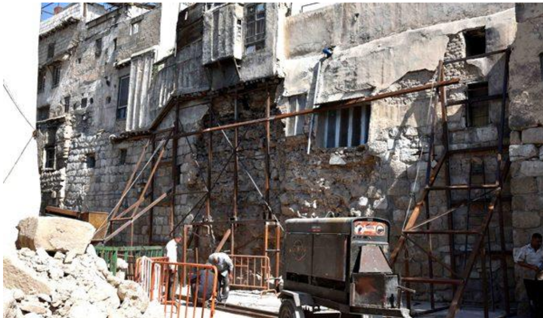
Figure 45: The renovation of the collapsed part of Damascus’s old city wall. The source: (Directorate of old Damascus, 2020).
