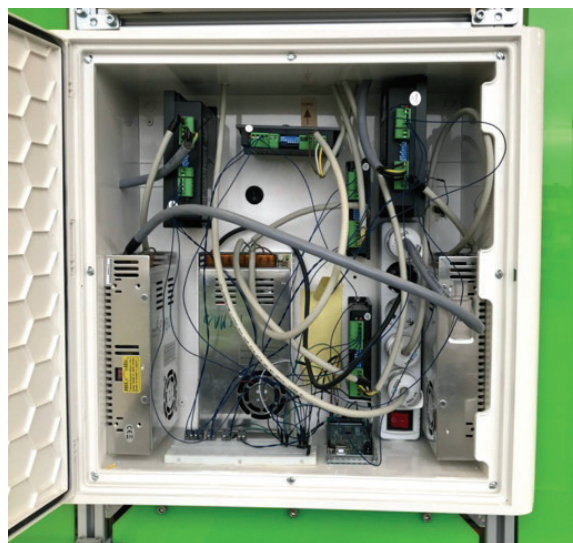
Figure 3.9. Electrical and electronic components of the machine.
