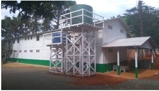
EXHIBIT 2 Use of elevated temporary reservoirs connected to the public water network [Color figure can be viewed at wileyonlinelibrary.com ]
