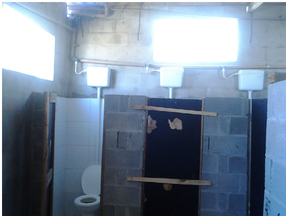
EXHIBIT 10 High-level flushing tank—site B [Color figure can be viewed at wileyonlinelibrary.com ]
