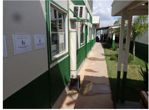
EXHIBIT 14 Collection of rainwater by the air-conditioning—site E [Color figure can be viewed at wileyonlinelibrary.com ]
