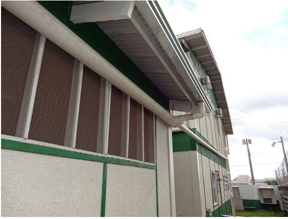
EXHIBIT 12 Rainwater harvesting by roof waterspouts—site E [Color figure can be viewed at wileyonlinelibrary.com ]
