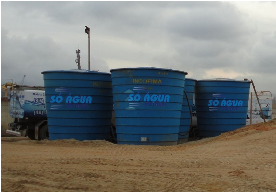
EXHIBIT 3 Use of temporary reservoirs supplied by the water truck. From: http://www.soaguapotavel.com/ [Color figure can be viewed at wileyonlinelibrary.com ]
