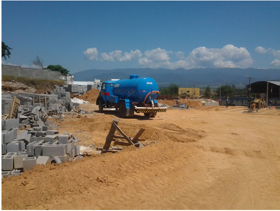
EXHIBIT 16 Water tanker vehicle to irrigate construction site—site B [Color figure can be viewed at wileyonlinelibrary.com ]
