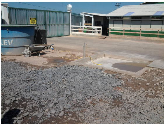
EXHIBIT 17 Place for washing vehicle wheels and concrete mixer truck with the metal hose—site E [Color figure can be viewed at wileyonlinelibrary.com ]
