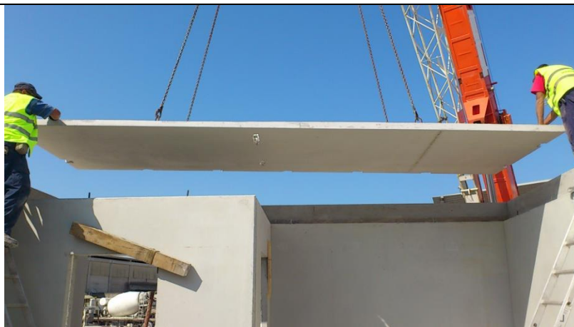
Figure 2: Details of construction system proposed: (a) internal view; (b) external view; (c) detail of cross-section with the wall supporting the slab; (c) placement of the pre-slab.
