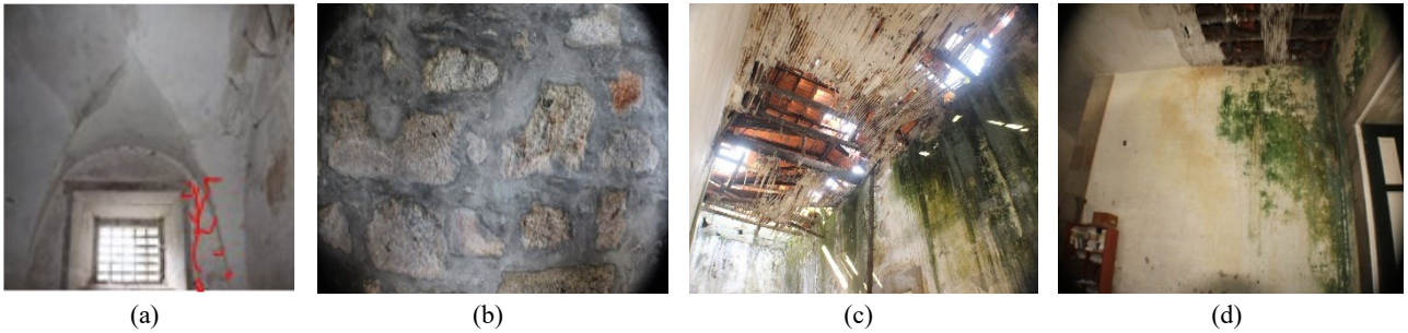
Figure 5: Damages. a) Cracks along the vault. b) Superficial alterations. c). Collapse of structural elements. d) Biologic colonization
