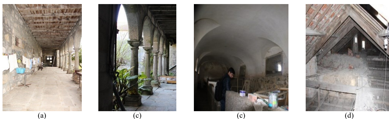
Figure 3: Structural typologies. a) Masonry walls and wooden floors. b) Granite stone pillars. c) Brick vaults. d) Wooden trusses.
