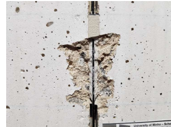
I-FA + CS Debonding at CFRP- Adhesive interface with concrete splitting
