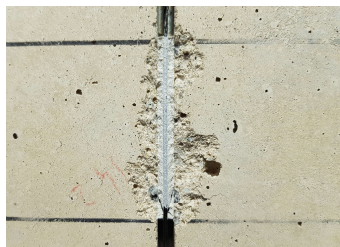
I-AC + CS Debonding at Adhesive- Concrete interface with concrete splitting
