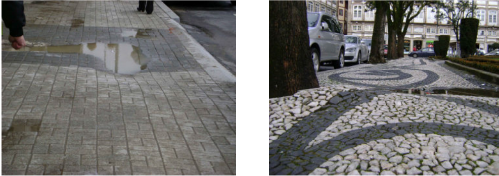
Fig. 6 Uneven Elevation of sidewalks in Guimarães City Center
