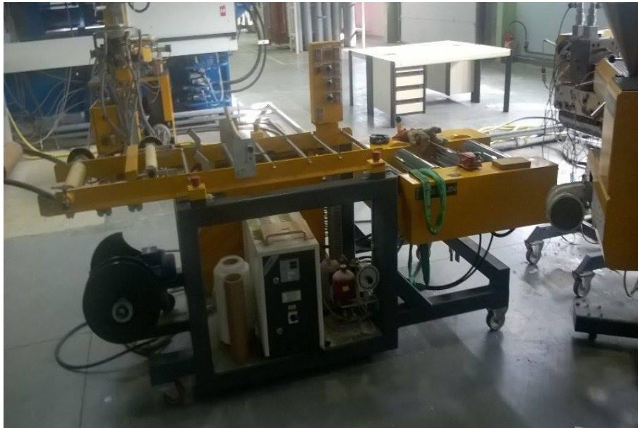
Figure 12 – Tearing and cooling system
