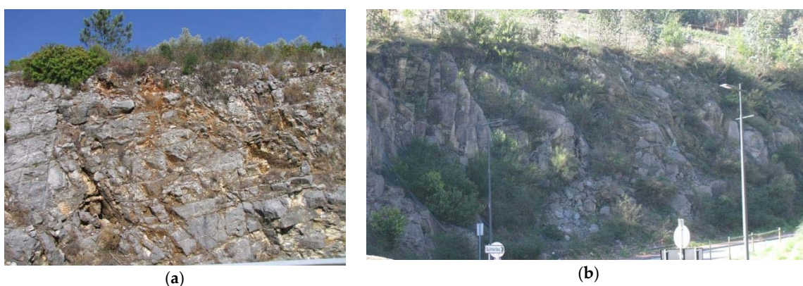
Figure 2. Stamps showing anthropogenic rock-cuts: (a) road slope on a limestone mass showing the bedding, joints and the effects of weathering (terra rosa); (b) road slope on a granite mass showing jointing that can promote rock movements, supporting net (to minimize this hazard) and natural recovery of vegetation.
