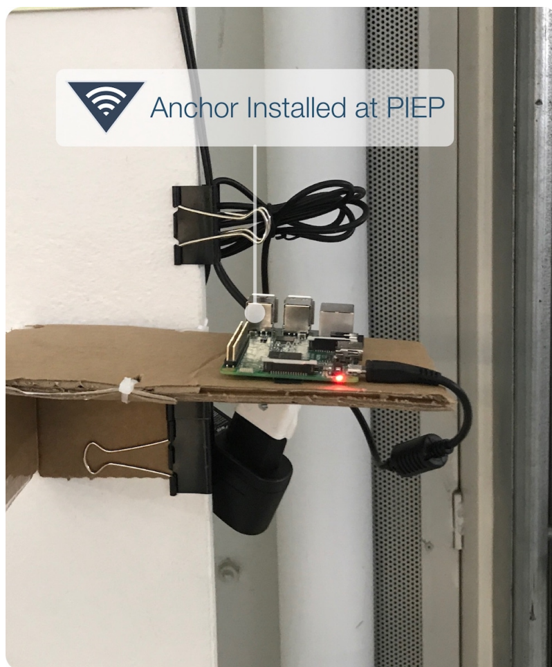
Figure 5.5: Photo of an Anchor at PIEP
