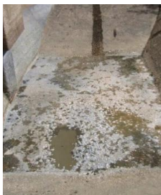
a) Abrasion in stilling basin
