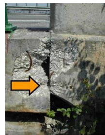
c) Crushed joints [8]
