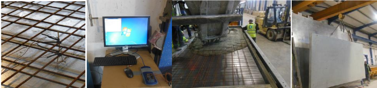
Figure 2: From left to right – Thermocouples attached on the reinforcement bars, temperature logging system, concrete wall casting on heating bed, wall lifted [photographs: F. Kanavaris].
