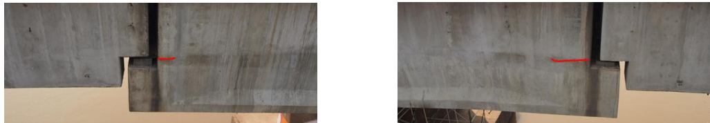
a) Cracks at Dechatiwong Bridge No.2 b) Cracks at Dechatiwong Bridge No.3
