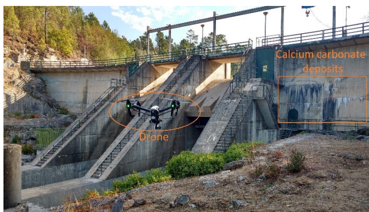
a) UAV (drone) visual inspection of dam with efflorescence ( \text{CaCO}_3 )
