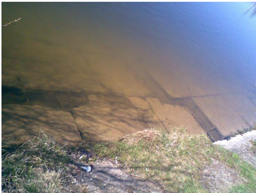
Figure 1: Destructed slabs for ponds slope protection in zone B.
