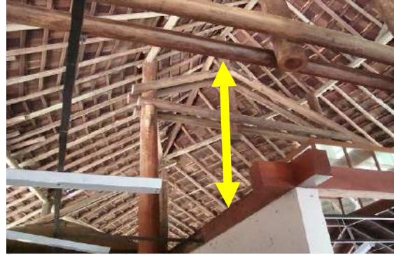
Photo 6 - the roof reaches a height up to 8 meters creating an air protection
