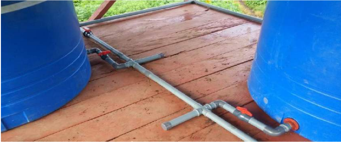
Figure 4. Interconnection of the water storage tanks
