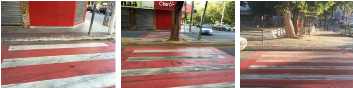
Figure 7: Lack of ramps to access sidewalks together with the pedestrian crossing.
