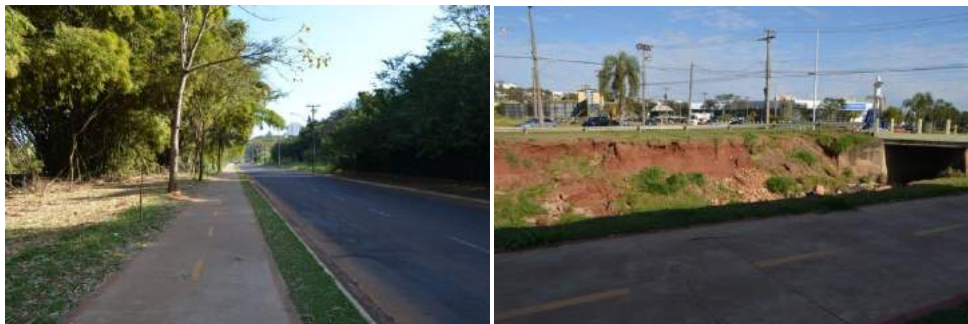
Figure 7. Francisco Pereira Lopes Avenue highlighting the bike path and landslip of the slope (photo on the right)
