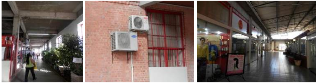
Figure 4: Ground Floor of the Municipal Market, with windows and a circulation corridor, improvised thermal conditioners installed on the facade of the building, facilities for sales stands of concrete and masonry, with a roof of metal structure, hollow elements and systems of air exchange.
