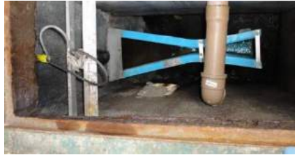
Figure 4. Parshall flume and ultrasonic level sensor
