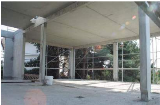
Figure 11. Subtle RC frame for energy efficient buildings used for construction of family house
