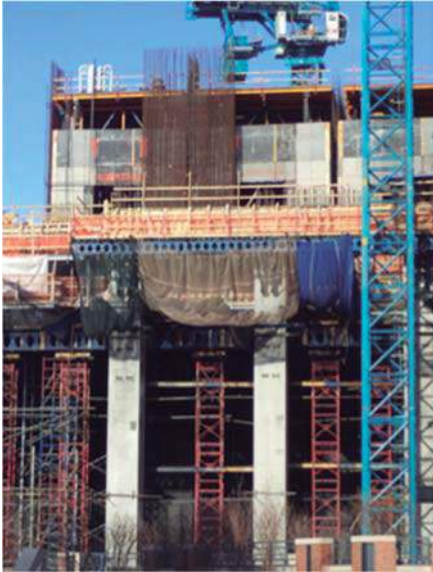
Figure 3. Strong impact in a construction site at the end of High Line, New York (Author: F. Muzzillo)
