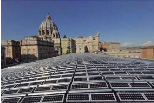
Figure 2 Photovoltaic panels in Vatican city (Inhabitat, 2014)
