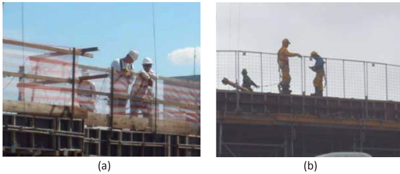
Figure 1. Example of compliance with TEPS requirements Both figures show workers supported on the TEPS, a frequent situation of use during the concreting stage.. (a) -WO. (b) TEPS-ME.
