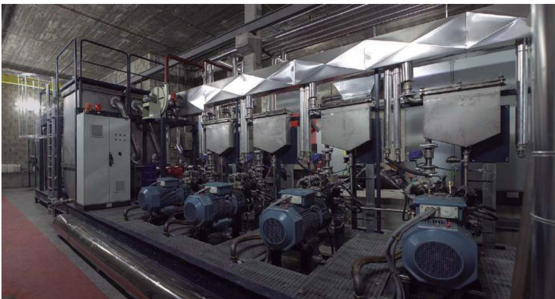
Figure 7. Biomass gasification plant
