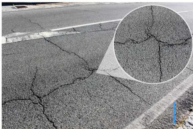
Fig. 2. Example of pavement with cracking.
