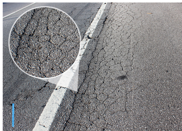
Fig. 1. Example of pavement with alligator cracking.
