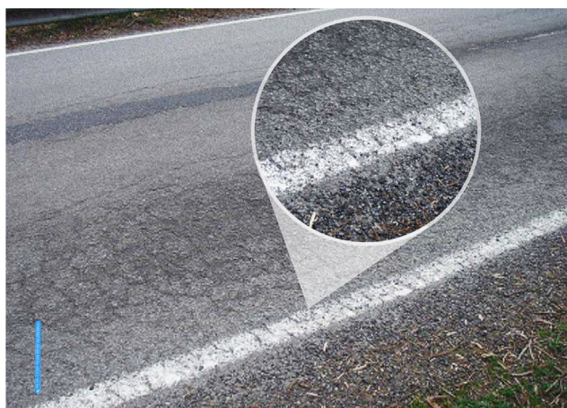
Fig. 3. Example of pavement with raveling.
