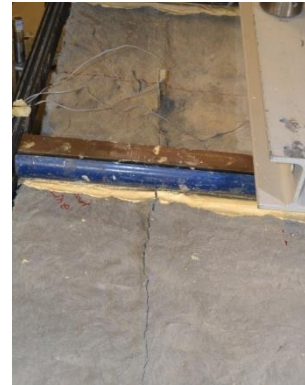
d) Splitting cracks in the DHCC layer in the alignment of the GFRP ribs
