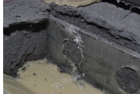
b) Compressive damage in the GFRP ribs
