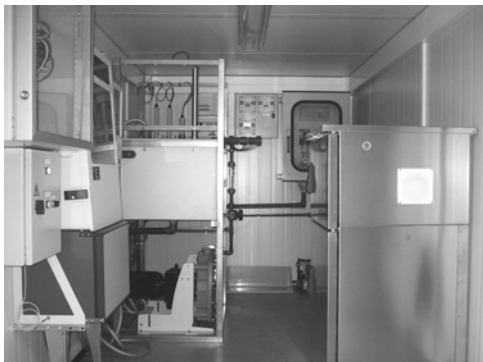
Fig. 2. On-line measurement station for eutrophication.
