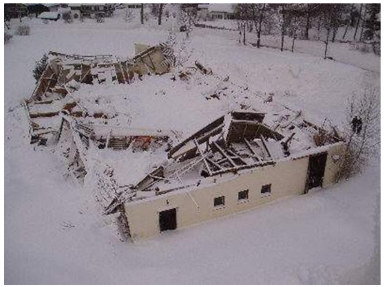
Roof failures under snow load Bavaria, 2006
