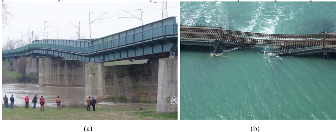
Figure 1 Failure due to scour – (a) pier settlement, Croatia 2009; (b) pier failure, Dublin 2009
