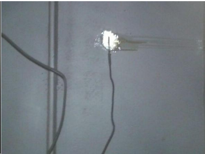
Welded strain meter
