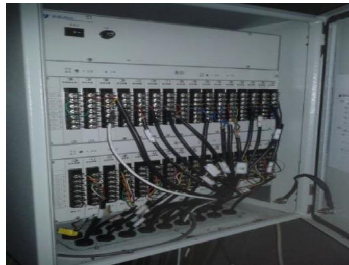
Data acquisition center
