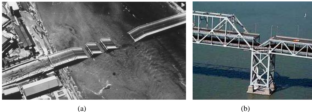
Figure 2 Failure due to seismic actions – (a) slab unsitting, Japan 1964; (b) slab unsitting, USA 1989
