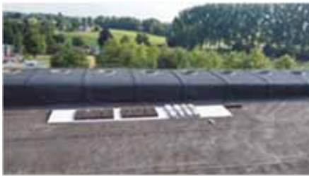
Figure 4 Natural ageing on the roof top of the BRRC building in Sterrebeek (Belgium).
