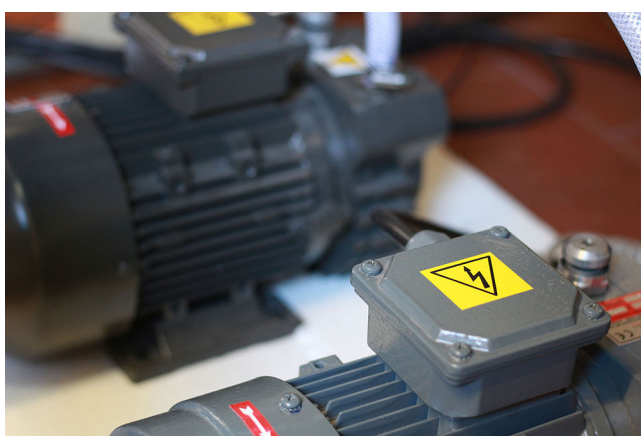
Figure 4.6: Vacuum system constituted by two GS-6 pumps in parallel
