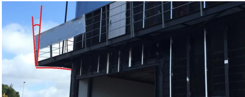
Figure 86 - Walkway needing renovation
