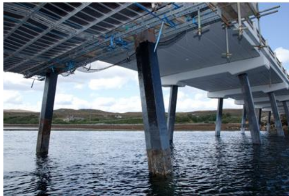
Figure 2. 15- Cathodic protection used in Kyle of Tongue Bridge [28]
