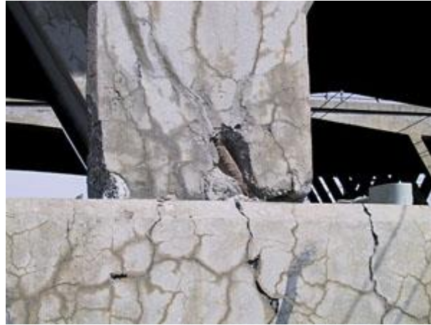
Figure 2. 12- Frost action damage in a reinforced concrete structure [26].
