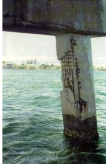
Figure 2. 11- Example of corrosion of reinforced concrete structures [24].
