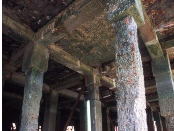
Figure 2. 14- Example of sulfate attack in a concrete structure near the sea. [25].
