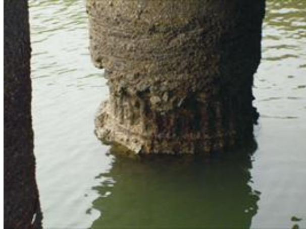
Figure 2. 13- Example of chloride attack in marine structures [24].
