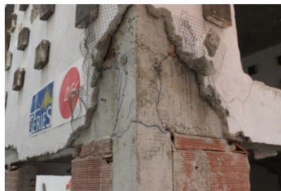
Fig. 16.12 Extensive cracking observed upon reinforced coating removal at the beam-column connection in the Northwest corner.
