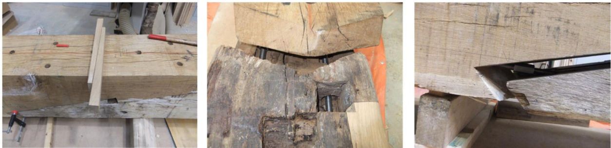
Fig. 24 – Scarf joint reinforced with glued in rods: steel rods are glued in both timber members and connected with a long nut (Credits: Pascal Lemlyn. Restauration du Moulin de l'abbaye de la Paix Dieu, Institut du patrimoine Wallon, Belgique).
