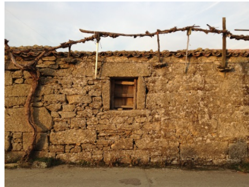
Figure 2. Green wall support system (corbels) on the masonry in Fariza de Sayago , Spain
