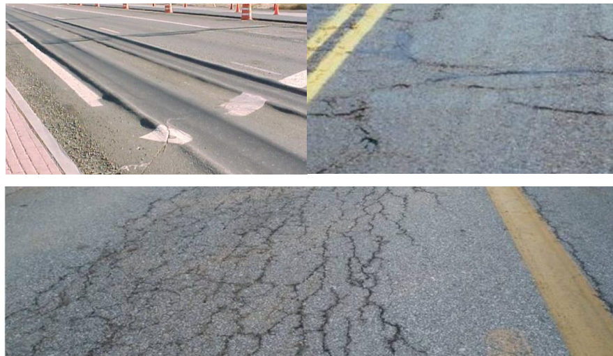
Figure 2-18 Representation of the different failures that road pavement undergo: rutting and cracking [27]
