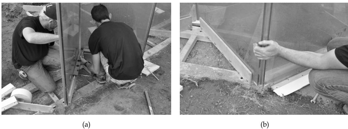
Figure 10.23. Verification of the angle between the panels (a) and fixing with the clamping profiles (b).
