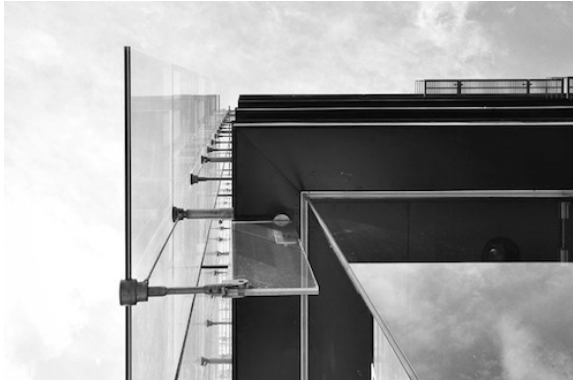
Figure 3.9. Close view of the connection detail between glass panel and glass fin of the Sendai Mediateque south facade.
