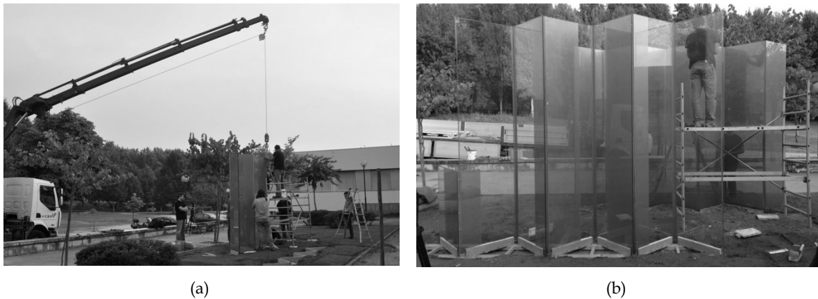
Figure 10.22. Placement of the panels in position using a crane (a) and assembly work of the second wall (b).
