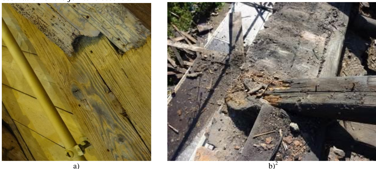
Fig. 1 Examples of degradation in trusses – a) wood element infested by wood-destroying insects, b) end beam rotted
