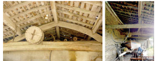
Figure 15. Examples of double and single pitched roofs. (Credits: C.E. Barroso et al.).
