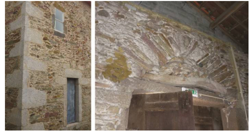
Figure 13. Examples of reinforced masonry walls with stoned worked granite and schist. Example of relieving arch. (Credits: C.E. Barroso et al.).
