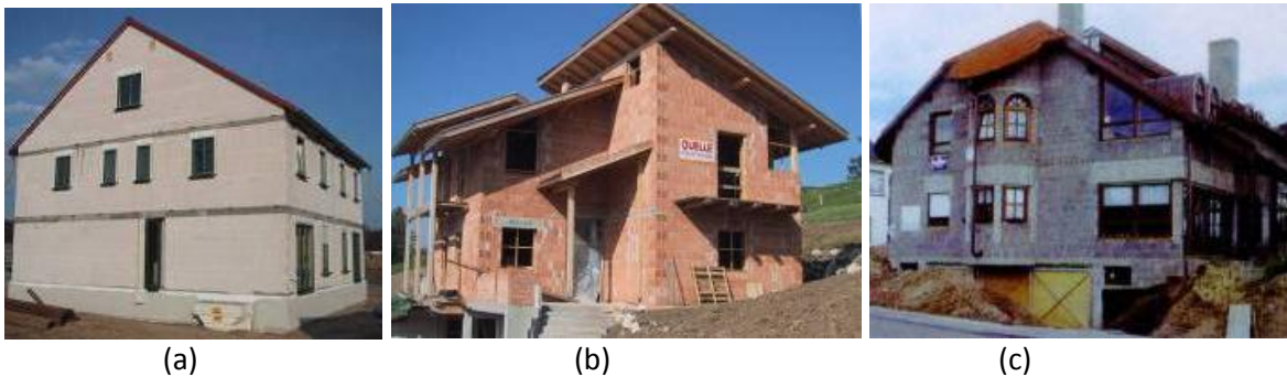
Figure 6. Modern unreinforced masonry integrated building systems; (a) calcium-silicate units; (b) clay units; (c) lightweight concrete units.
