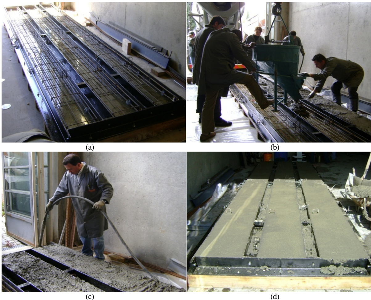
Figure 3.17: Slab strips specimens: formwork setup (a), concrete casting (b), concrete vibration (c) and final aspect of the slab strips (d).
