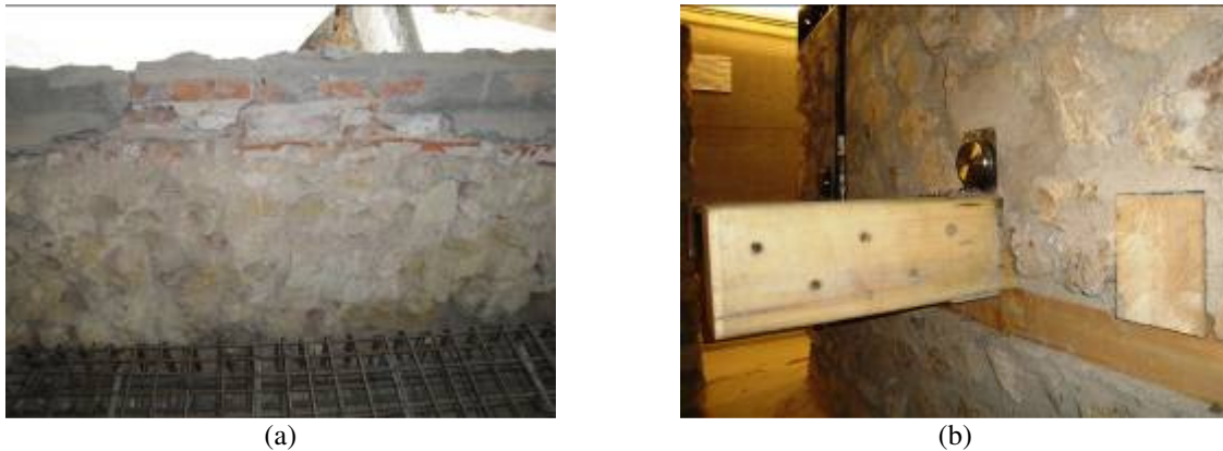
Figure 2 Masonry wall: (a) from a 'Pombalino' building; (b) detail of the connection built in the laboratory
